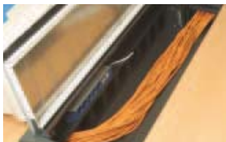
Intelligent cable management in spacious cable ducts.
