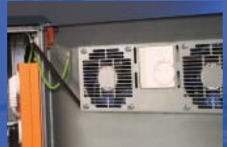
Power distribution and ventilation
