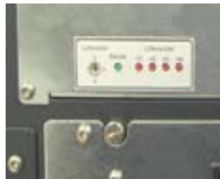
Fan failure display/ four speed levels
